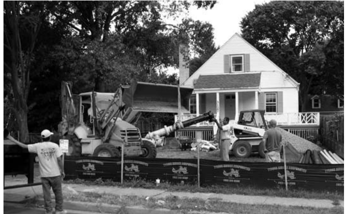
The Total Development Solutions crew prepares the building site for Doorways' future Freddie Mac Foundation Family Home. The existing structure is slated to be demolished in late September.
